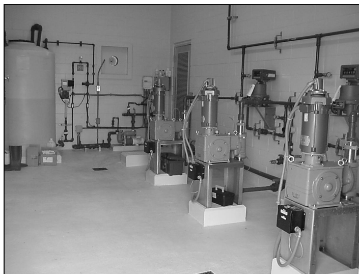
Figure 6.1 Alum Treatment System and Injection Equipment
