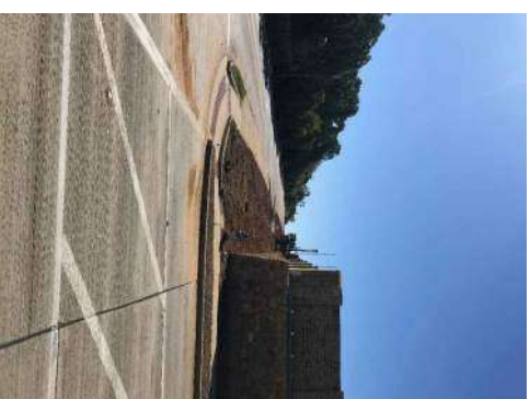
WALL ENCROACHMENT (LOOKING SOUTH ALONG TOWER RIDGE DRIVE)
