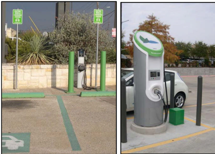
Figure 11: An EV Charger is not required to be installed for EV Parking Spaces
