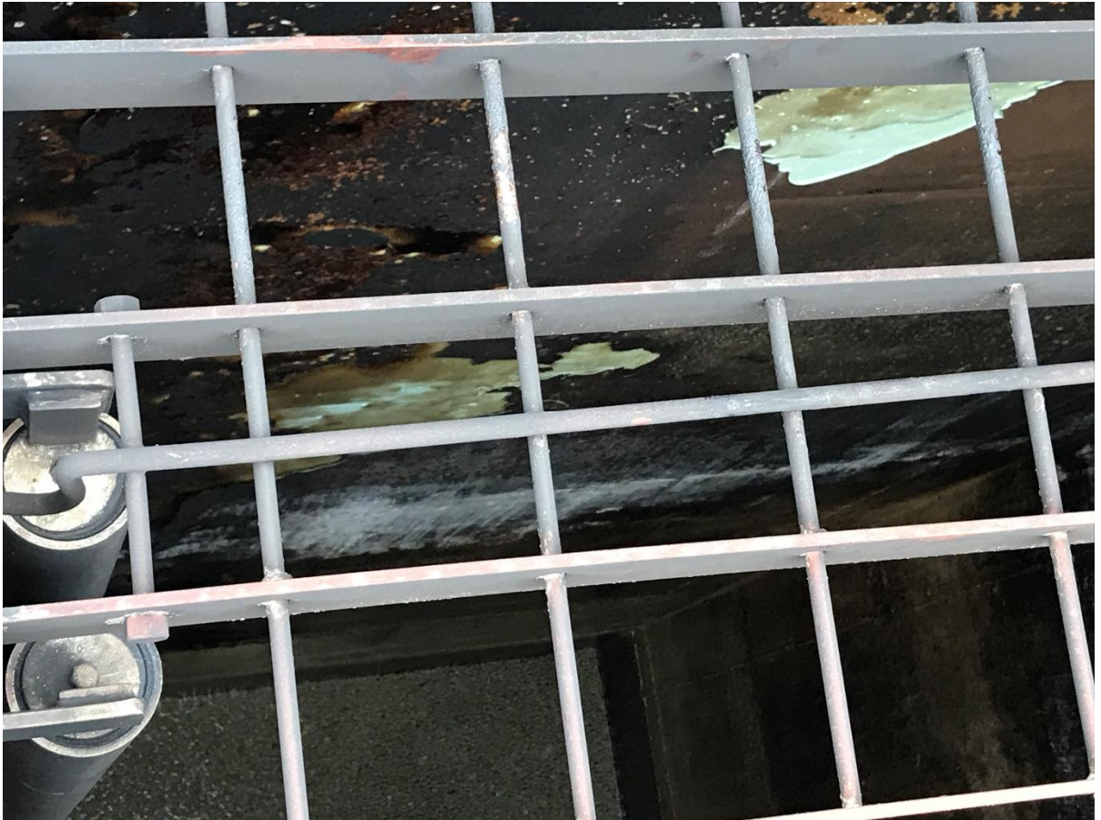
Damaged Wet Well Coating
