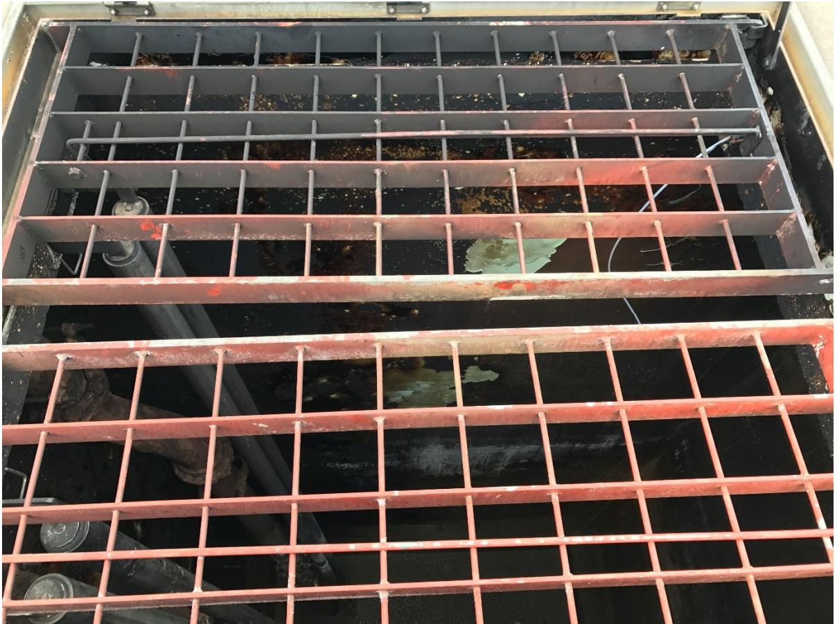
Damaged Wet Well Coating
