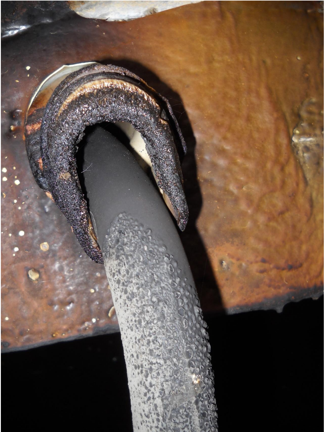
Pump #3 – Damaged Cable Jacket and Conduit
