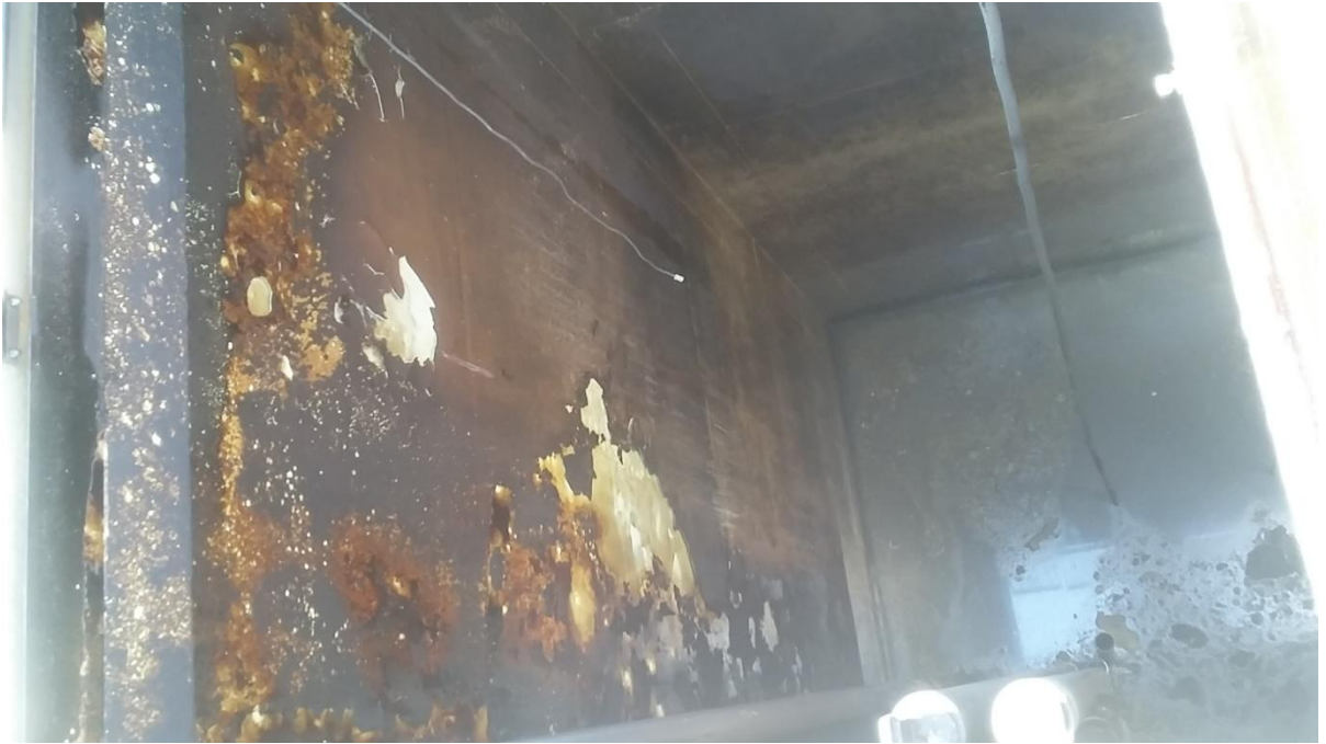
Damaged Wet Well Coating
