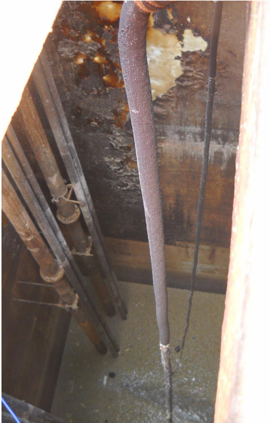
Pump #2 – Damaged Cable Jacket
