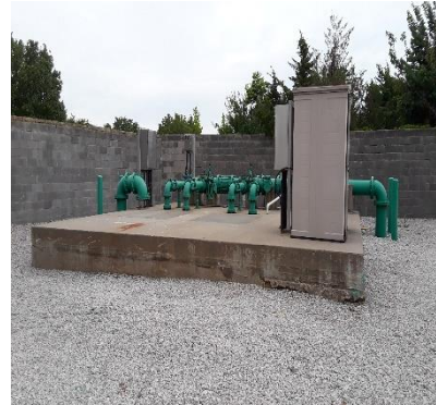
13 Sanitary Lift Stations Maintained
