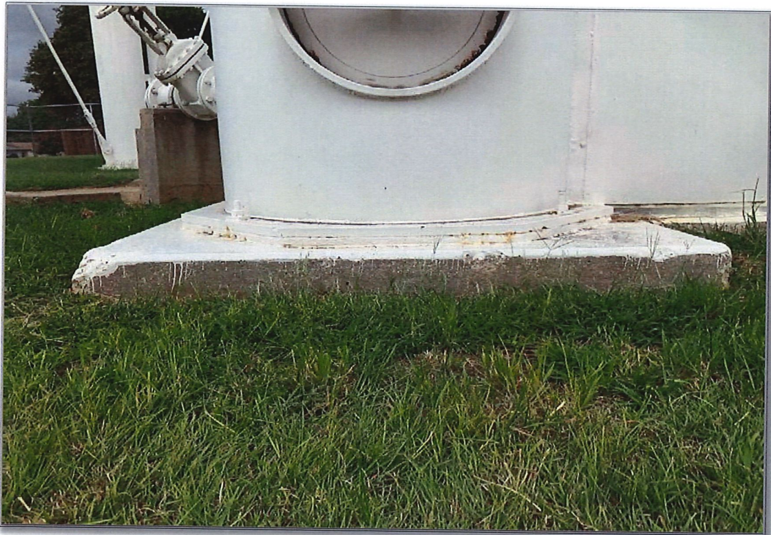
6) TOWER RISER AT GROUND SURFACE
