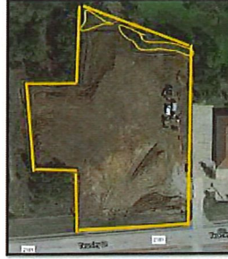
FM2181 just east of Acme Brick west of Parkridge Drive
